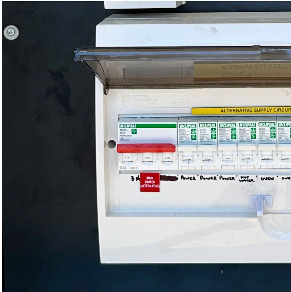
Figure 3: Compliant - labelling of “MAIN SWITCH – ALTERNATIVE” at a load centre.
