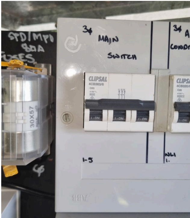
Figure 3: Non-compliant switchboard with no “MAIN SWITCH (GRID)” label.
