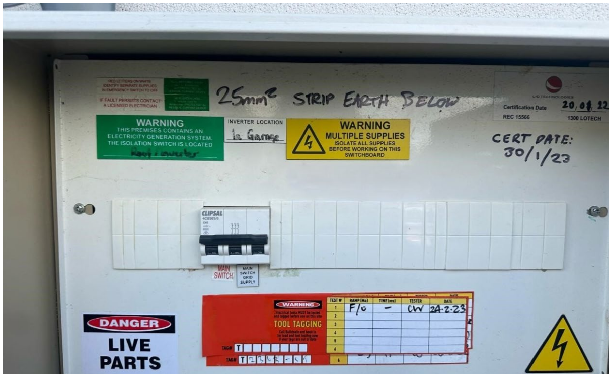
Figure 3: Incorrect 'Multiple supplies' label applied.
