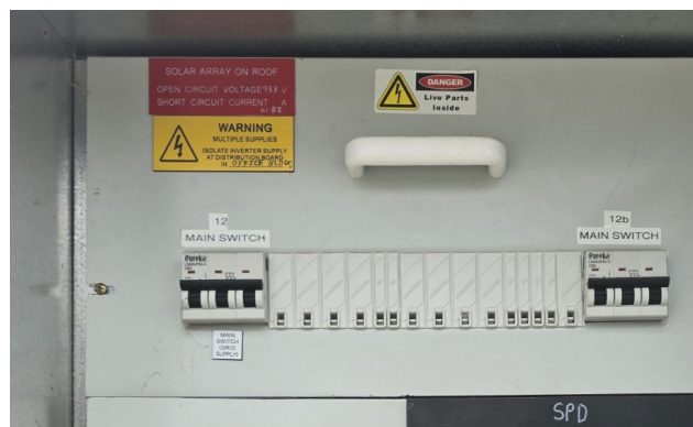
Figure 1: 'Warning Multiple Supplies' label has been compliantly installed at the MSB indicating the location of the distribution board to isolate the inverter supply.
