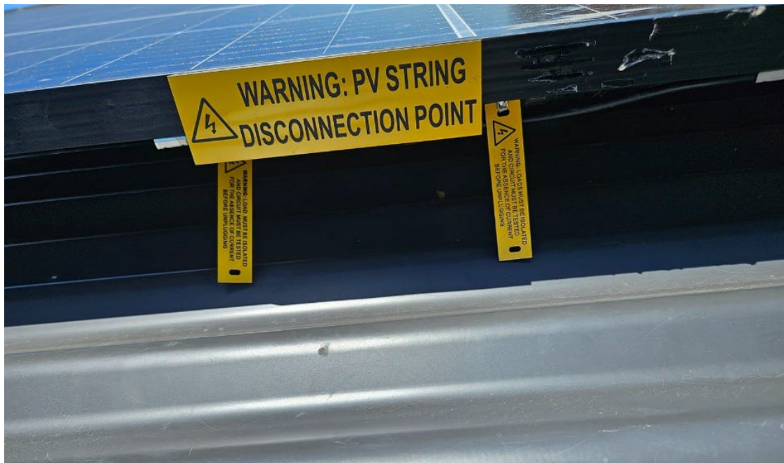
Figure 5: Compliant warning label placed within 300mm of the two disconnection points.
