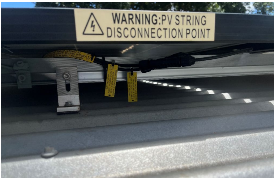
Figure 4: The disconnection point is fixed to the rails greater than 300mm from the warning label, this is non-compliant.
