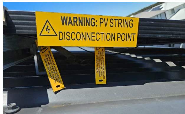
Figure 1: Compliant warning labels placed within 300mm of the disconnection point.
