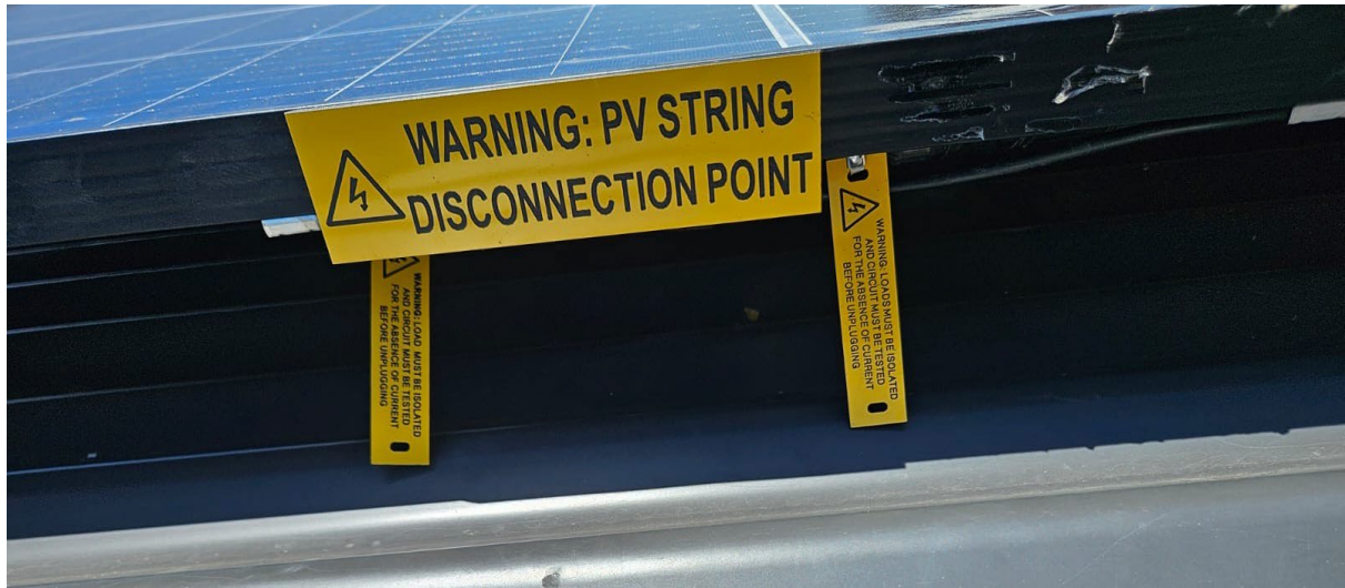
Figure 5: Compliant Labels correctly applied to both the positive and negative cable within 100mm of the disconnection point using stainless steel ties. Labels are UV stable and engraved.
