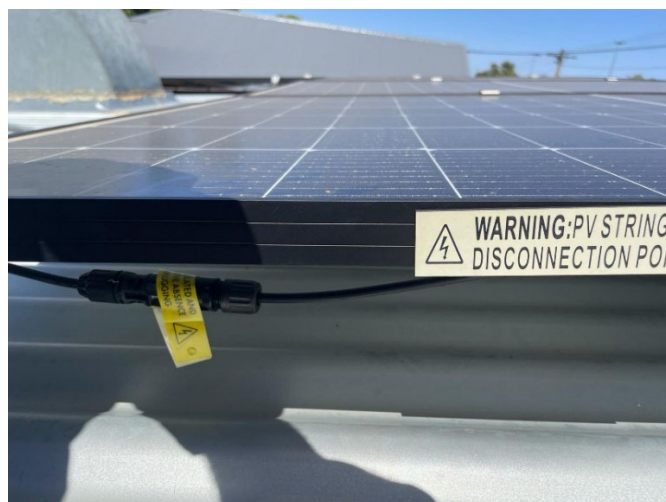
Figure 4: With one label across the disconnection point and the label not durable for the location, this is non-compliant.
