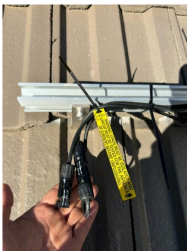
Figure 3: One label used across both conductors, fixed with plastic ties, this is non-compliant.
