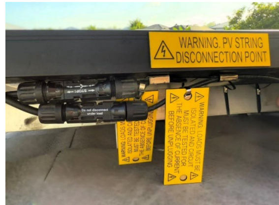
Figure 1: Compliant Warning labels applied to both positive and negative cables within 100mm of the disconnection point, using stainless steel ties.
