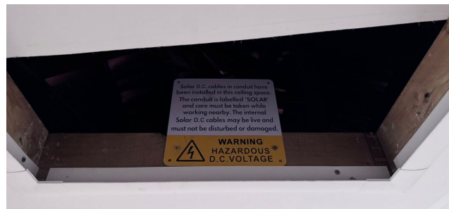
Figure 1: A compliant label installed adjacent to the access point of an accessible roof space.
