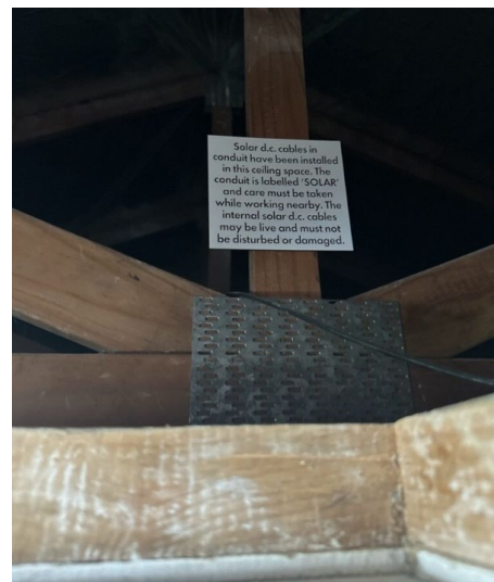
Figure 3: Non-compliant: the label does not contain the WARNING: HAZARDOUS d.c. VOLTAGE portion of the label.
